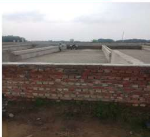
Distribution of gravel in Sludge Drying Bed
