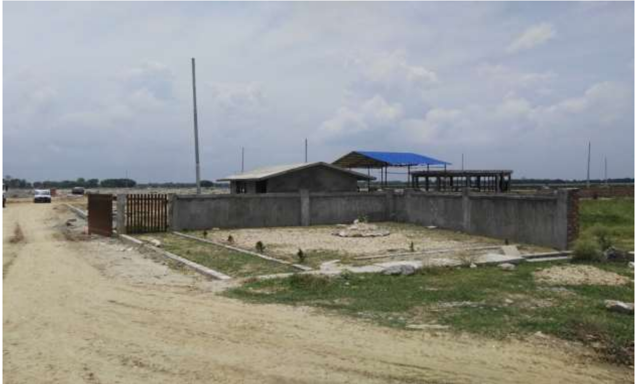
A view of WWTP, Jatuwa from the entrance gate
