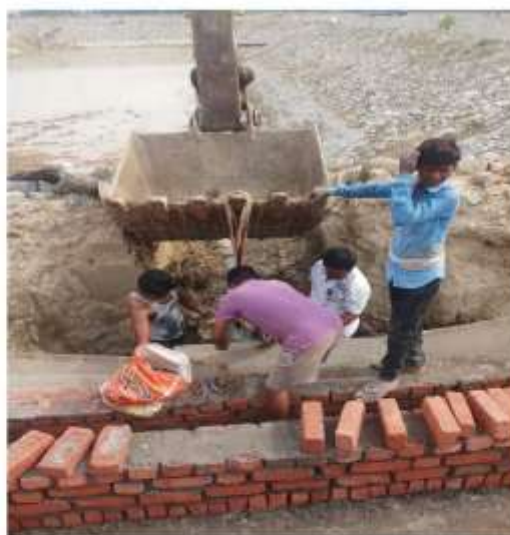
Pipe Valve Fitting in Pipe Inspection Chamber
