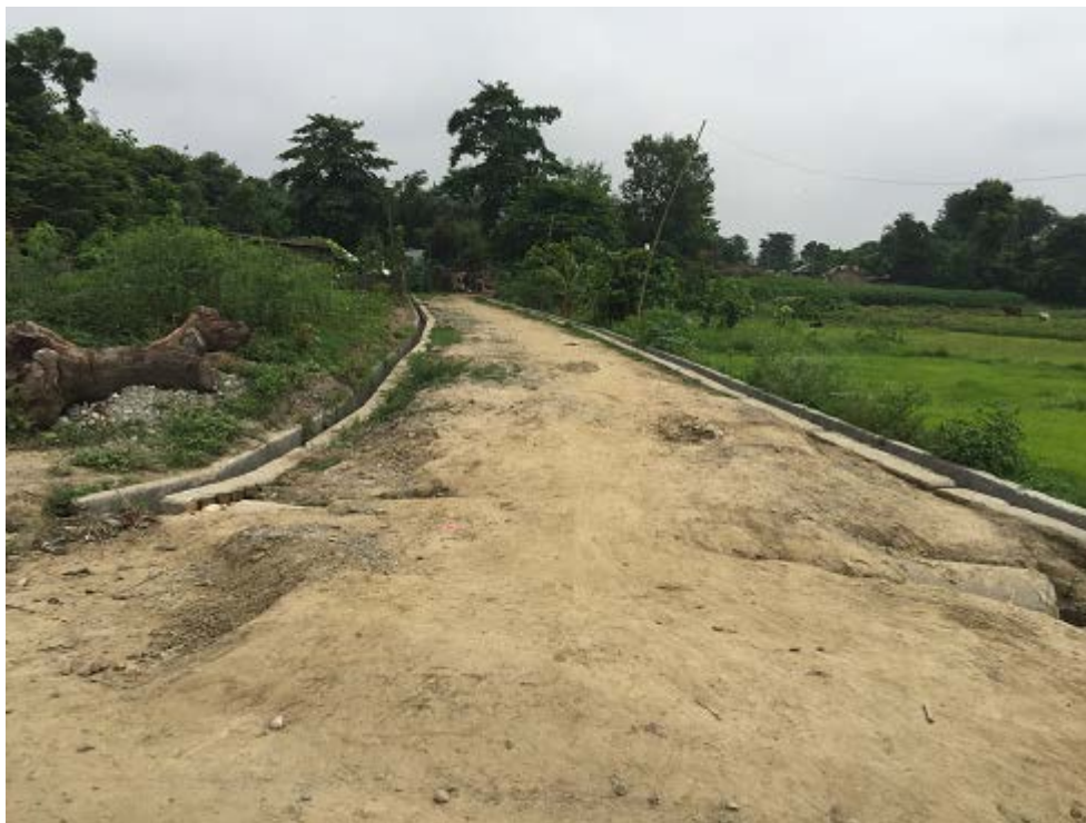
Figure 1. Pending gravel works due to scarcity of construction materials
