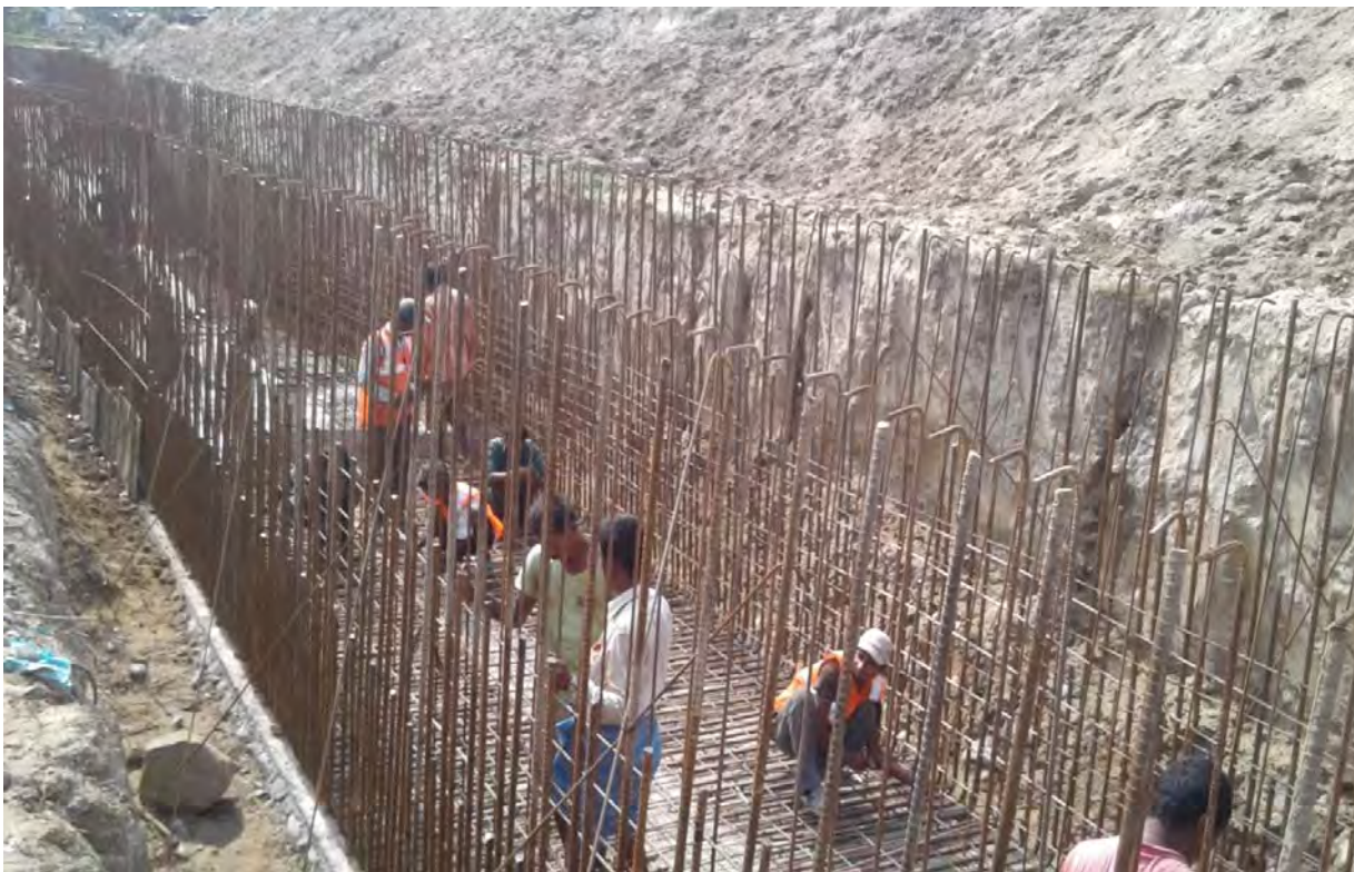
Storm water drain at A1
