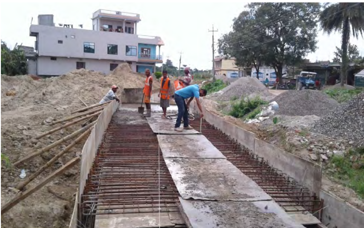
Storm water drain at A1
