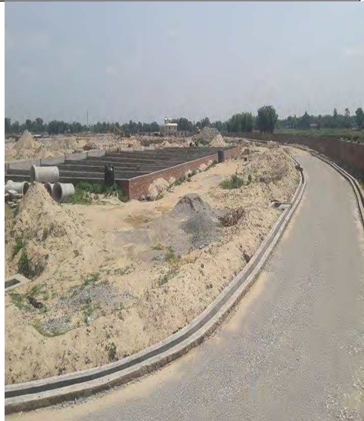
Sludge Drying BED
