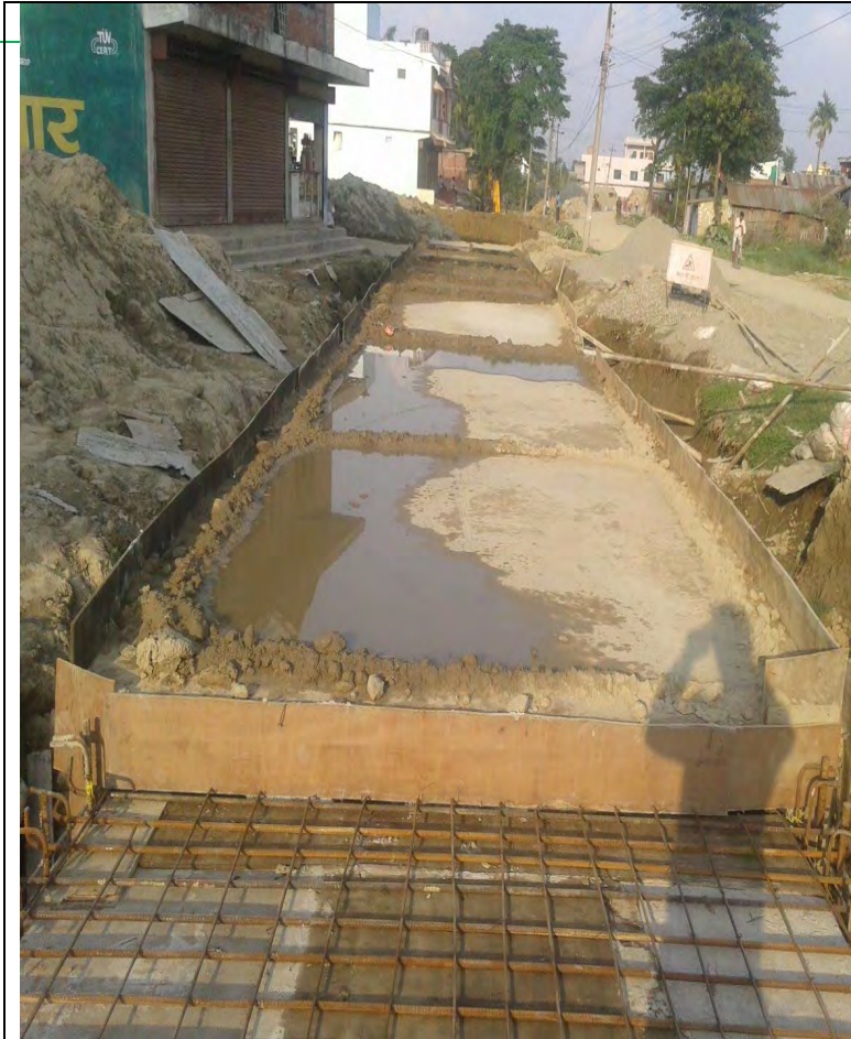
RCC Storm Drain at Line A1L2
