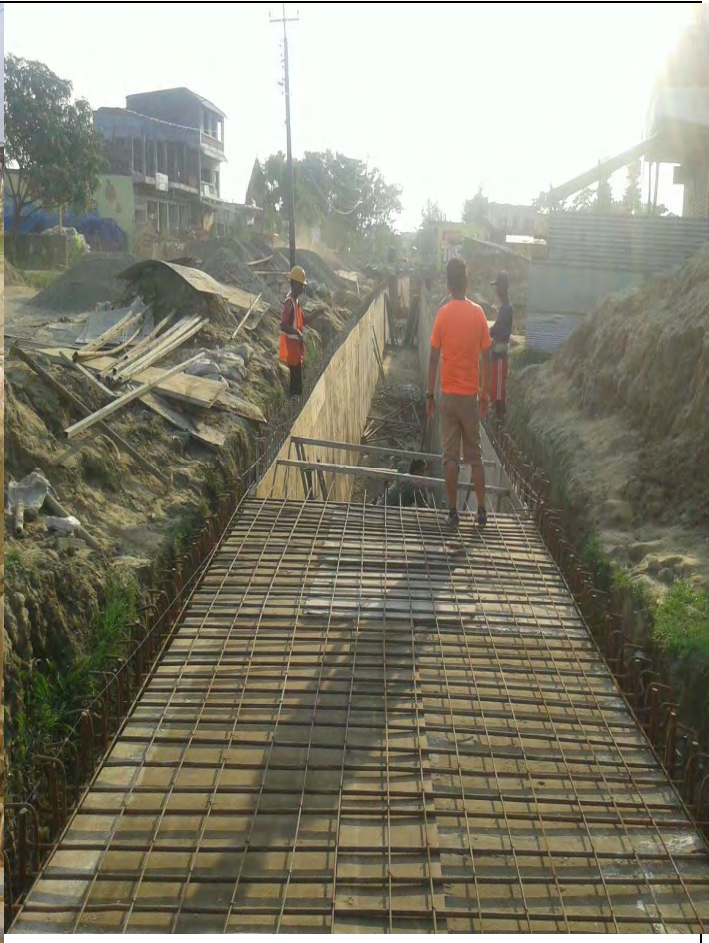
RCC Storm Drain at Line A1L1
