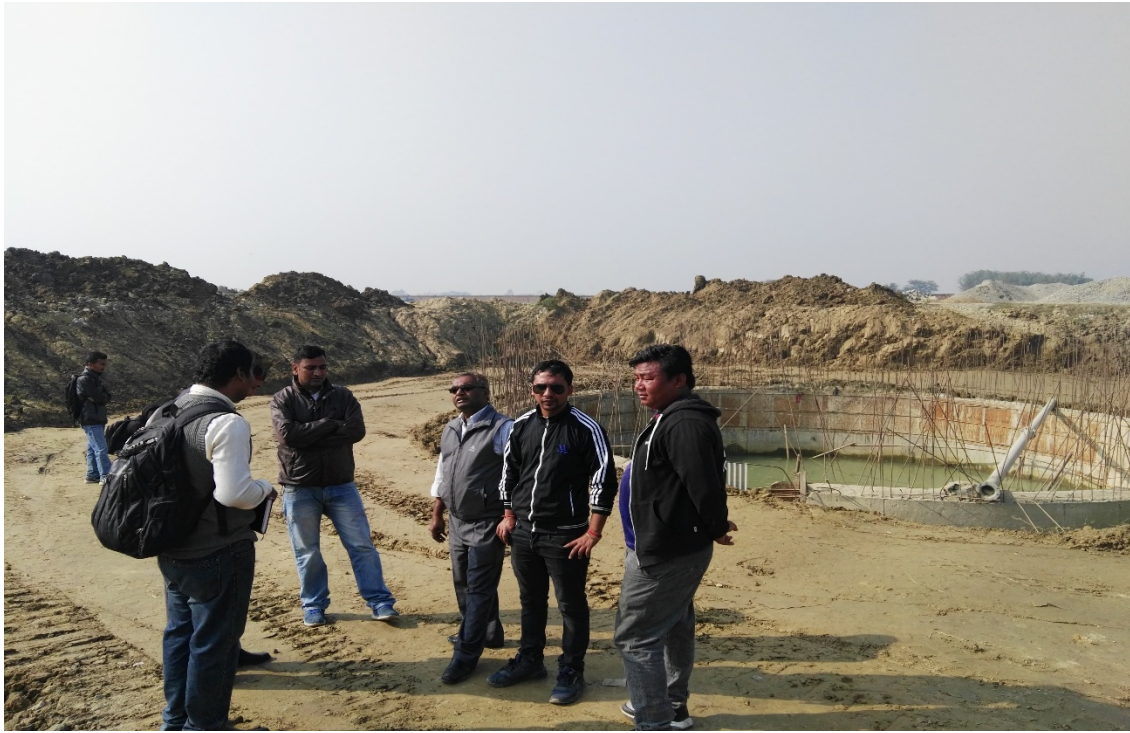
A view of Sump Well at WWTP
