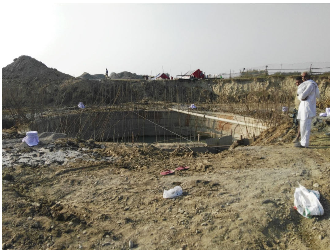
A view of Sump Well at WWTP (after creation of six bore holes)
